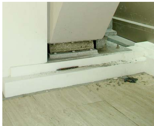
Figure 12 -- Photo of the beam center pad at the long span beam above the isolated side stage
