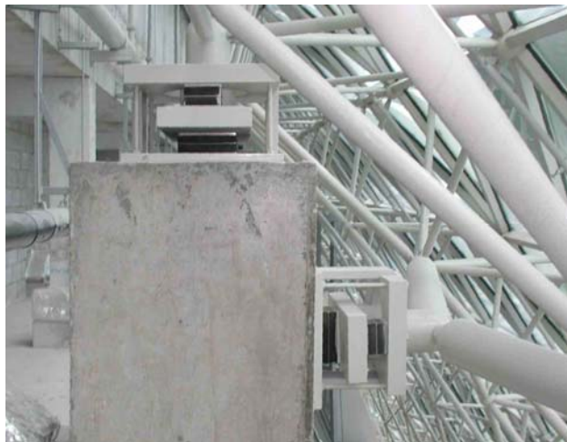
Figure 11 -- Roof structure double acting rubber isolator assemblies at the Esplanade performance halls
